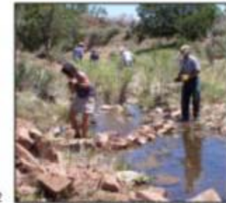
Rock Baffle Before
